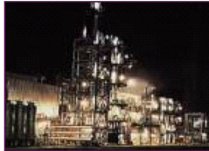
SCGP demonstration plant Harburg 150 tpd
