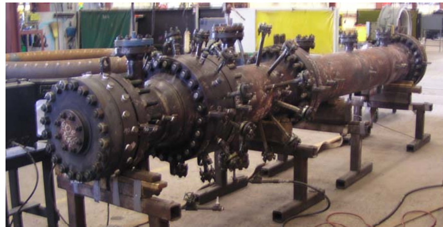
Gasifier and Quench Hardware Assembly
