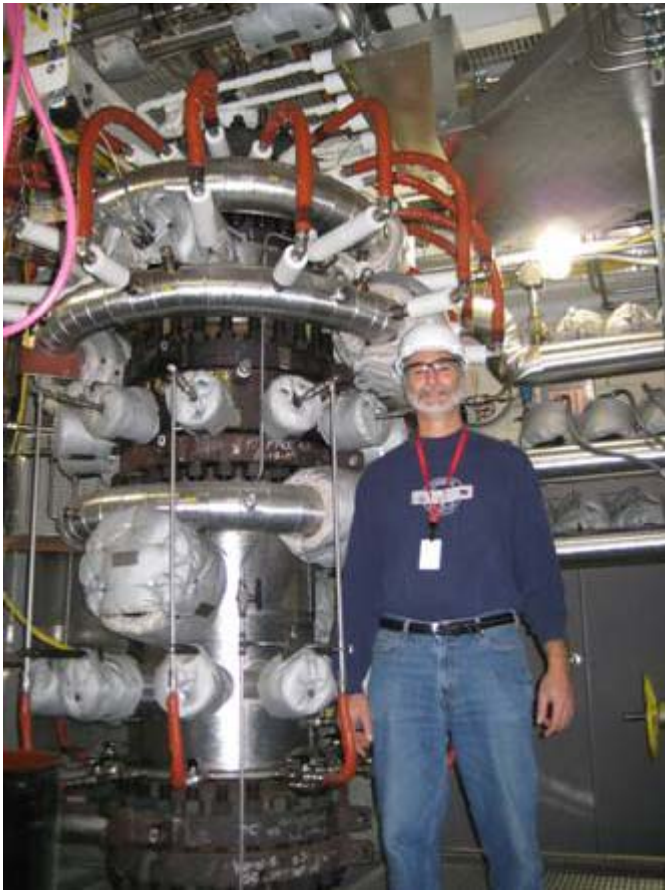
Gasifier installed in process bay at GTI
